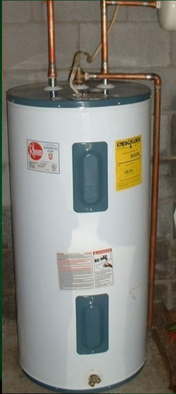
Electric hot water tank
